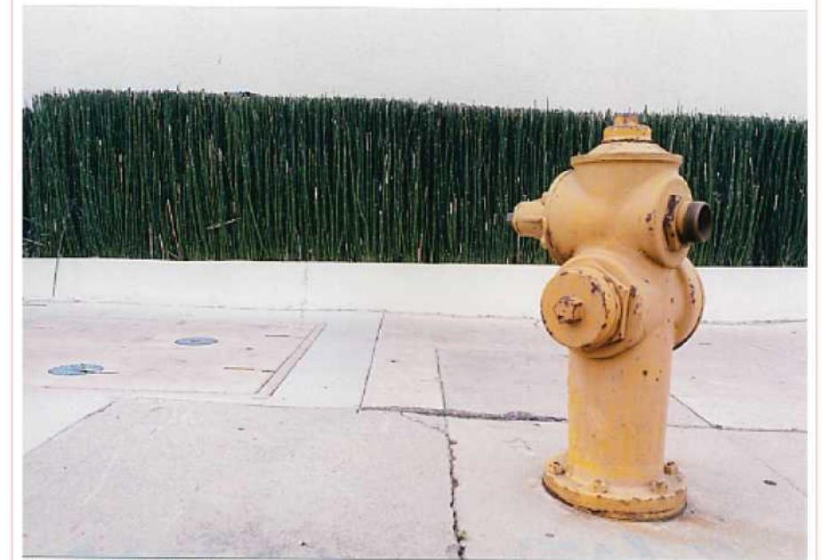
Fire hydrant in Los Angeles.
