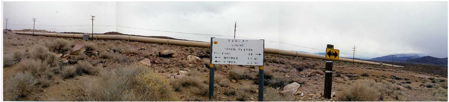
Pipeline delivering water along alternate route to three power stations along the 3,000 foot deep Owens River Gorge.
