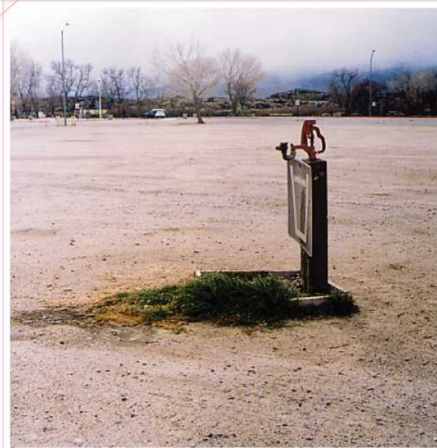
RV water refill station at a rest-stop on Highway 395.
