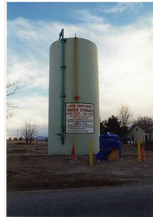
Emergency water storage, Laws.
