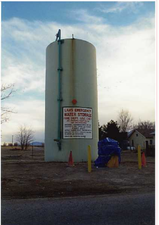
Fire emergency water tower, Laws.
