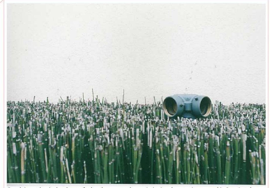
Standpipe pokes its head out of a bamboo grass planter, imitating the vegetation around it. Los Angeles.
